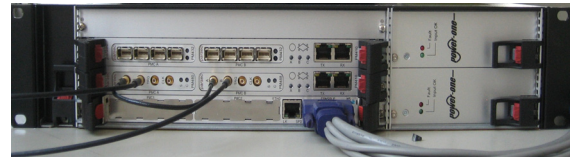
Figure 8: Signal processing system.
